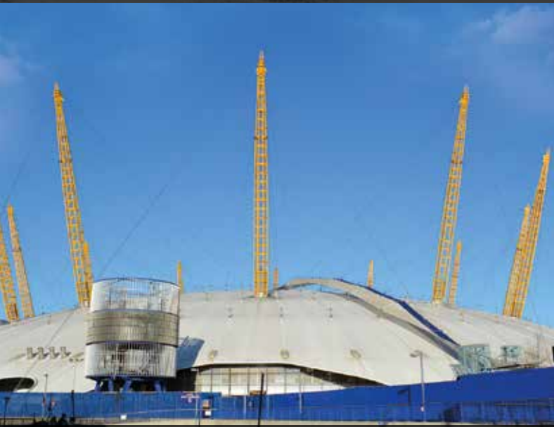
INSTALLATION: O2, LONDON
